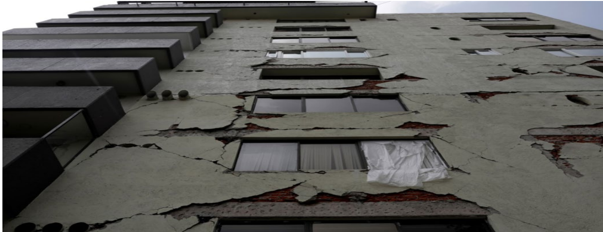
Photo 1 - Building damage from the 2017 Mexico City Earthquake
