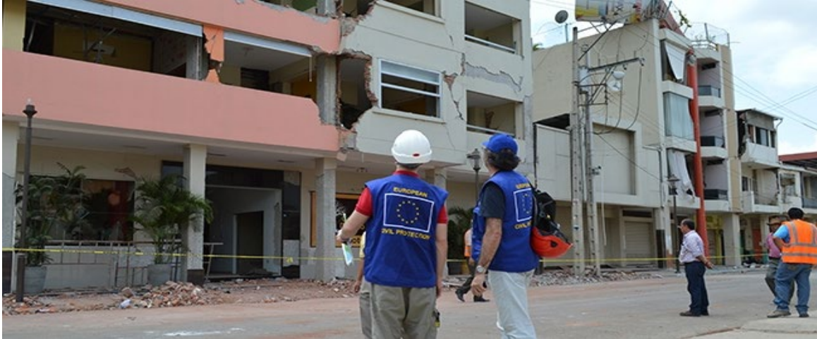
Photo 2 - Engineers inspecting a building damaged from an earthquake
