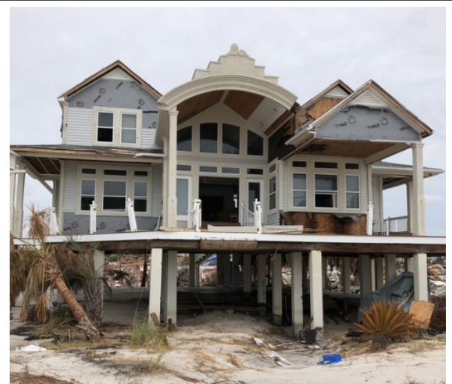
Figure 9. This home, built in 1997, did not have enclosed areas under the elevated floor. Mexico Beach after Hurricane Michael (Prevatt).
