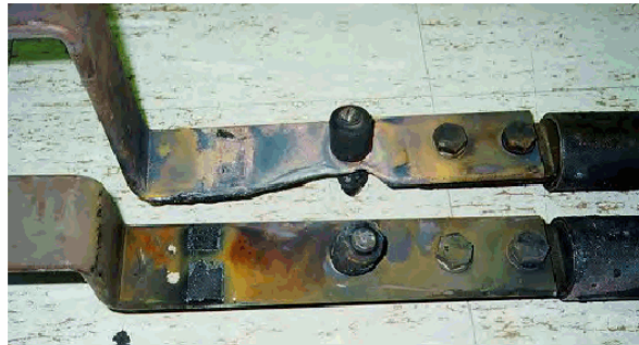
Figure 2-5 Copper Busbar Melted by Surge Current
