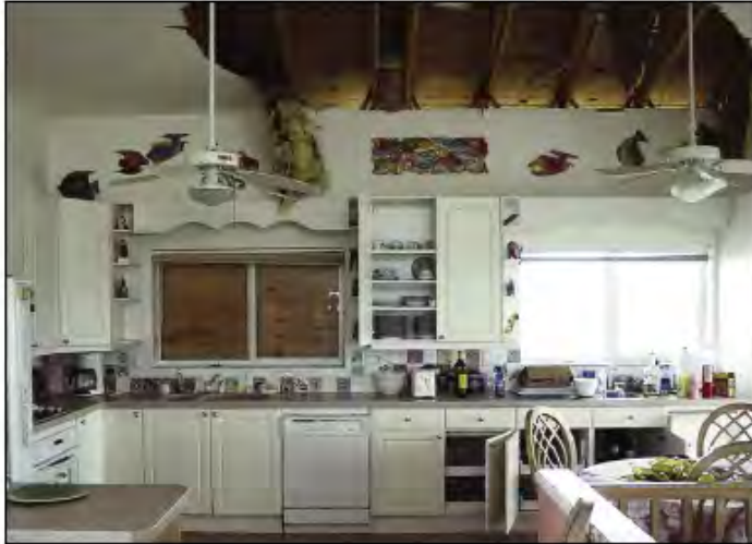
Figure 3-22. The drywall ceiling in the home shown in Figure 3-21 collapsed after becoming waterlogged and weakened by wind-driven rain that entered through the exterior soffit space. Plywood covers the opening of a window broken by windborne debris after the plastic shutters blew off (North Captiva Island).
