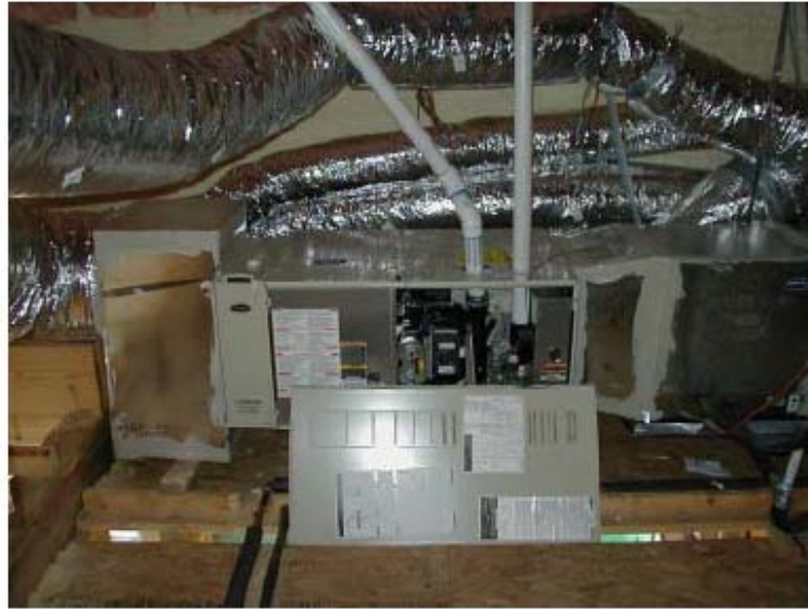
Figure A-6a. Photograph of air handler unit of two-stage compressor with ECM fan and Thermidistat system
