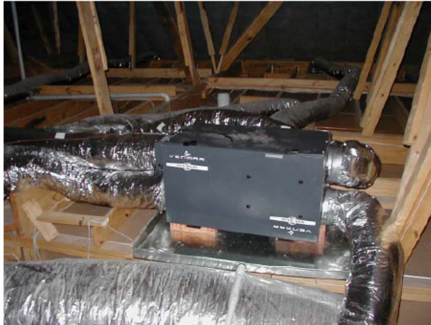
Figure A-5a. Photograph of ERV system located in conditioned attic
