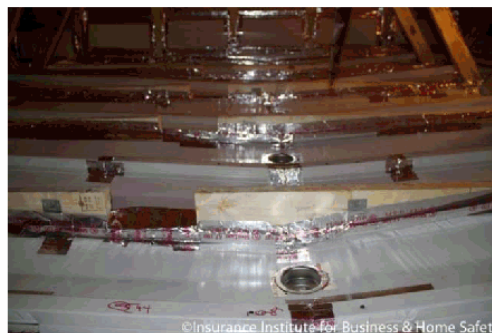
Figure 3 - Photograph of water collection channels between ceiling trusses in duplex.
