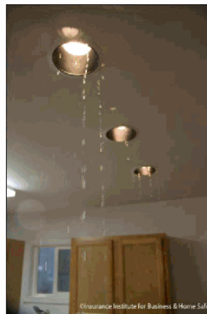
Figure 10 - Photograph of the water entry during the demonstration event on the un-sealed roof deck side of the duplex: close up of the recessed lighting in the kitchen.
