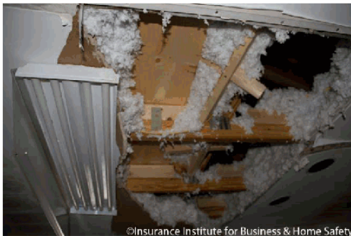
Figure 12 - Photograph of collapsed ceiling in the kitchen on the un-sealed roof deck side of the duplex.
