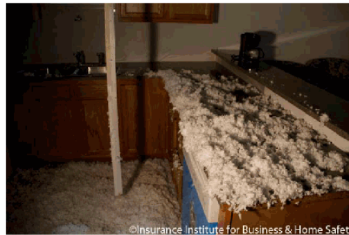
Figure 13 - Photograph of fallen portions of collapsed ceiling in the kitchen on the un-sealed roof deck side of the duplex.
