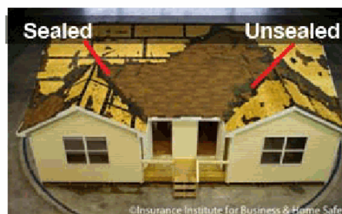
Figure 9 - Photograph of the front of the duplex after shingle and underlayment removal using high winds, illustrating the sealed roof deck (on the left) and the un-sealed roof deck (on the right).
