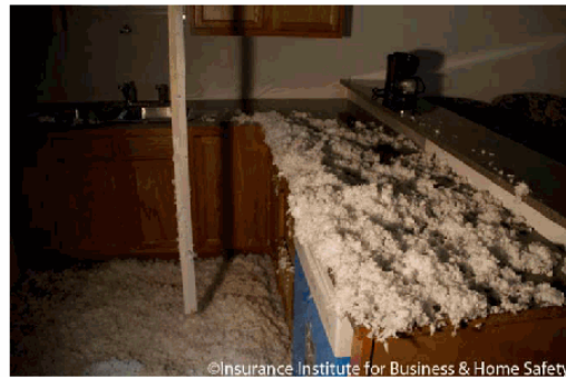
Figure 13 - Photograph of fallen portions of collapsed ceiling in the kitchen on the un-sealed roof deck side of the duplex.
