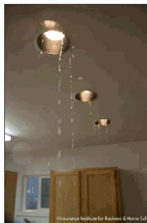
Figure 10 - Photograph of the water entry during the demonstration event on the un-sealed roof deck side of the duplex: close up of the recessed lighting in the kitchen.
