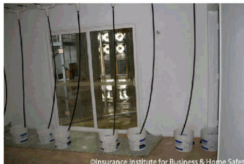
Figure 5 - Photograph of water collection drains to collection buckets in the duplex.
