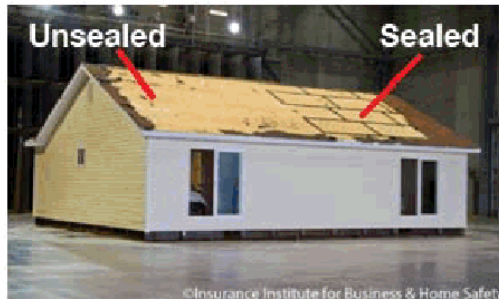
Figure 8 - Photograph of the back of the duplex after shingle and underlayment removal, illustrating the sealed roof deck (on the right) and the un-sealed roof deck (on the left).
