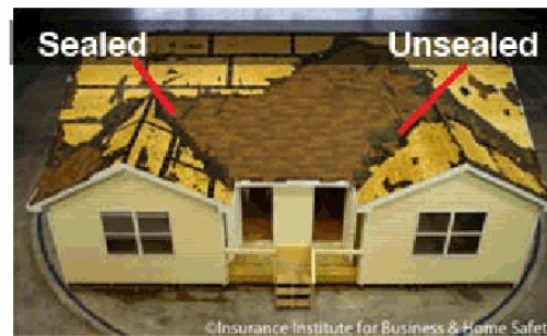
Figure 9 - Photograph of the front of the duplex after shingle and underlayment removal using high winds, illustrating the sealed roof deck (on the left) and the un-sealed roof deck (on the right).
