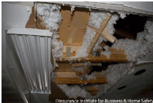
Figure 12 - Photograph of collapsed ceiling in the kitchen on the un-sealed roof deck side of the duplex.
