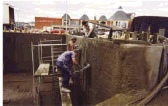
Figure 2: Use of mechanical screed and finishing machine. It took a crew of three craftsmen about an hour to finish the wall.
