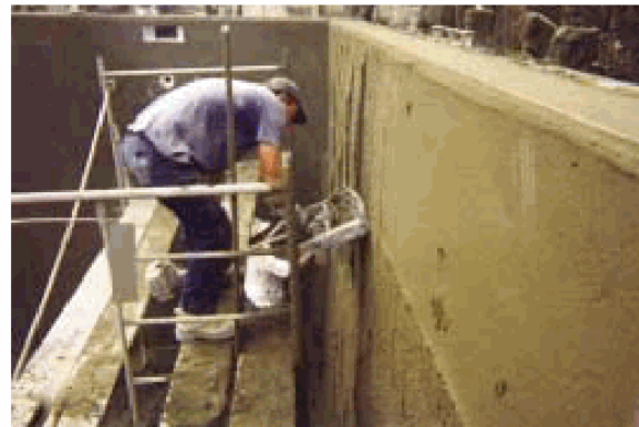
Figure 3: Close-up of the screeding device. Note the wall in the background, made of one monolithic layer of shotcrete and fully finished (no plastering needed).
