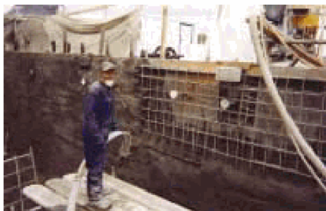
Figure 1: Example of steel layout for a pool being constructed in the city of Quebec. Note the two layers of #10M steel (between US#3 and US#4) spaced at 8 in. (200 mm) in both directions.
