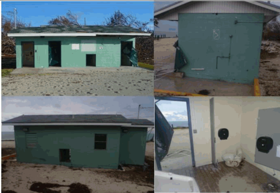
Figure 5. Florida, after Hurricane Irma, flood Zone V. No evidence of structural damage after estimated 5 ft stillwater plus waves. From upper left: facing beach, side, interior, rear.
