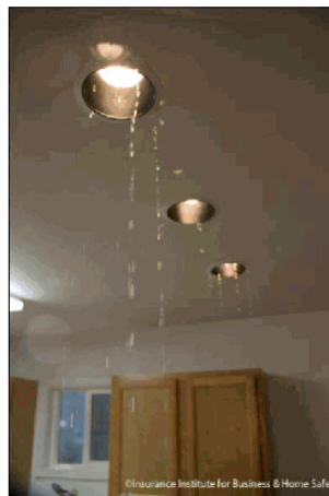
Figure 10 - Photograph of the water entry during the demonstration event on the un-sealed roof deck side of the duplex: close up of the recessed lighting in the kitchen.
