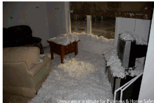
Figure 14 - Photograph of fallen portions of collapsed ceiling in the living room on the un-sealed roof deck side of the duplex.
