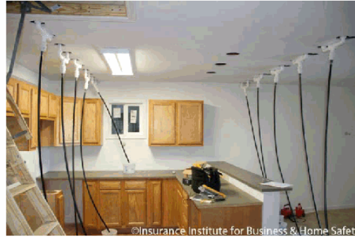
Figure 4 - Photograph of water collection drains to collection buckets in the duplex.
