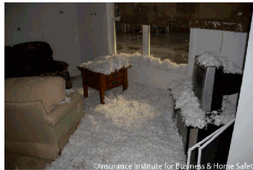
Figure 14 - Photograph of fallen portions of collapsed ceiling in the living room on the un-sealed roof deck side of the duplex.
