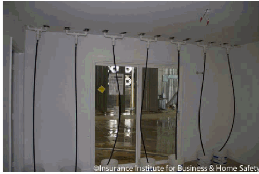
Figure 6 - Photograph of water collection drains to collection buckets in the duplex.
