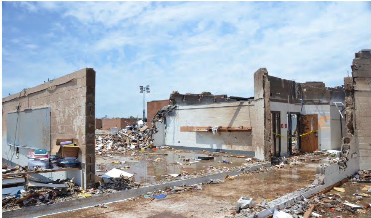
Figure 1. Damage to the New Main Classroom Building at Plaza Towers Elementary School. The seven schoolchildren died in the central hallway when the classroom walls collapsed on them. An additional two staff members and one student were injured in this building.
