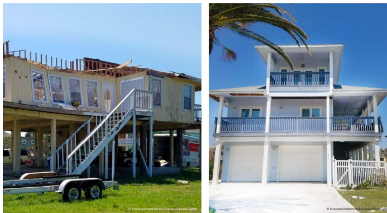
Figure 24. Comparison of two homes located 250 ft apart that experienced similar wind speeds during hurricane Harvey (2017) but performed very differently in Port Aransas North. The older construction was built in 1987(left), and newer construction was built in 2006 (right).
