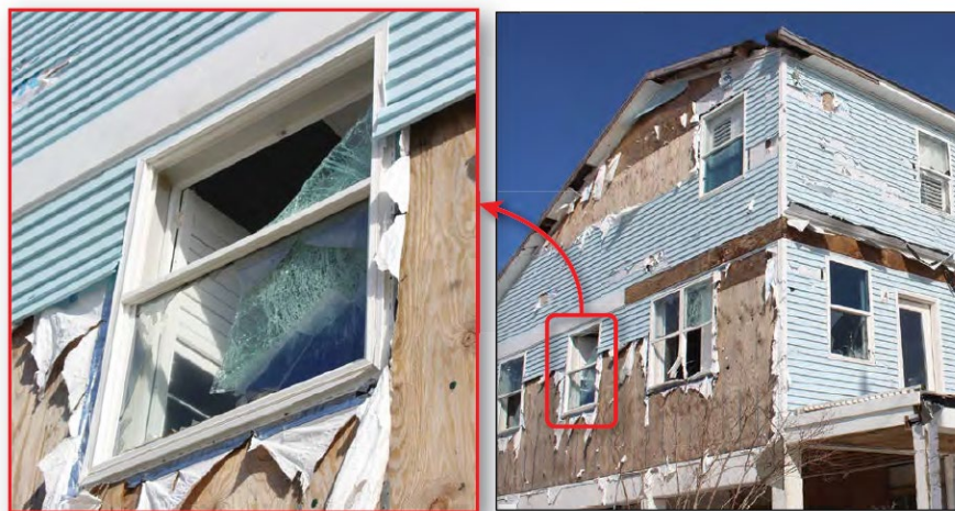
Figure 29. Impact resistant window after Hurricane Michael (2018) in a house built in 2010, located in Mexico Beach. Estimated wind speeds (150 mph) exceeded the design wind speeds (130 mph).
