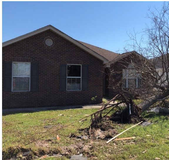
Figure 36. Damage to a window cause by wind-borne debris in Panama City during Hurricane Michael (2018). House was built between 2000-2009 and located 3.27 miles from St. Andrew Bay. Estimated wind speeds (129-150 mph) might have exceeded the design wind speeds (135 mph).
