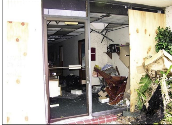
Figure 15. Broken windows in an office caused by Hurricane Charley (2004) in Punta Gorda.
