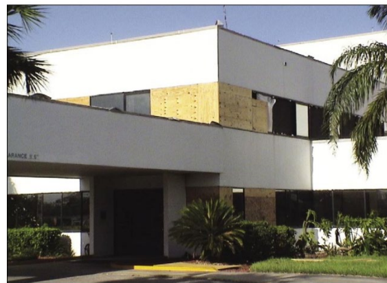
Figure 12. Damage in the windows in a hospital in Arcadia during Hurricane Charley (2004). EWS = 110-120 mph.
