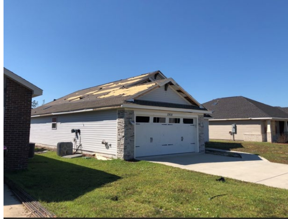
Figure 35. Damage to a garage door in Panama City during Hurricane Michael (2018). House was built between 2000-2009 and located 3.39 miles from St. Andrew Bay. Estimated wind speeds (129-150 mph) might have exceeded the design wind speeds (135 mph).
