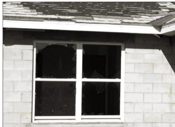
Figure 17. Broken window by wind-borne debris during Hurricane Charley (2004), in Deep Creek.
