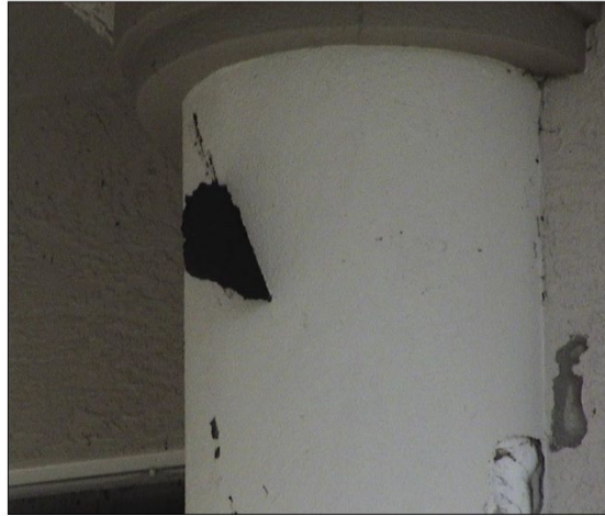
Figure 8. Asphalt shingle on a column in Punta Gorda during Hurricane Charley (2004)
