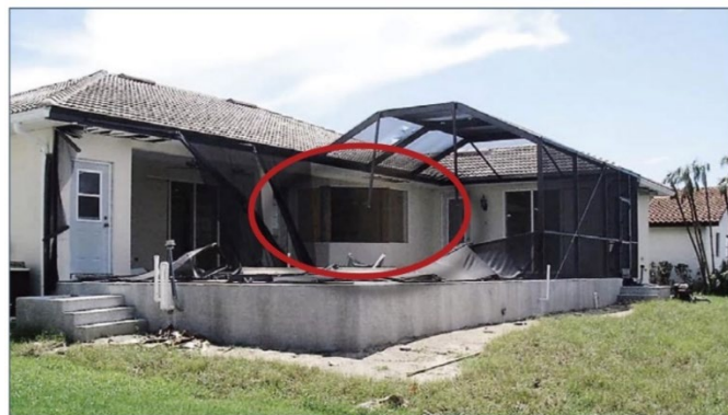
Figure 14. Broken window from debris (in the red circle) caused by Hurricane Charley (2004), in Punta Gorda.
