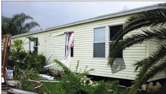
Figure 16. Windows broken in a manufactured home by wind-borne debris during Hurricane Charley (2004) at the east of Port Charlotte.
