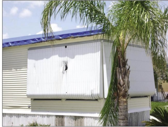
Figure 18. Metal awning shutter penetrated by a missile in Zolfo Springs during hurricane Charley (2004).
