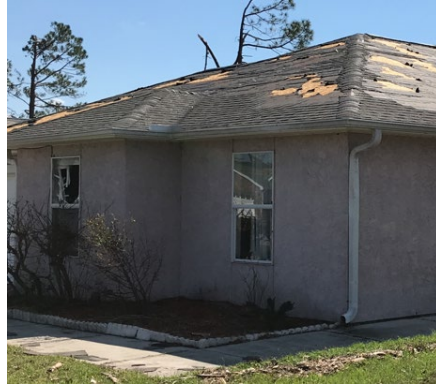
Figure 37. Damage to windows in a hose located in Panama City during Hurricane Michael (2018). House was built between 1990-1999 and located 3.25 miles from St. Andrew Bay. Estimated wind speeds (129-150 mph) might have exceeded the design wind speeds (135 mph).
