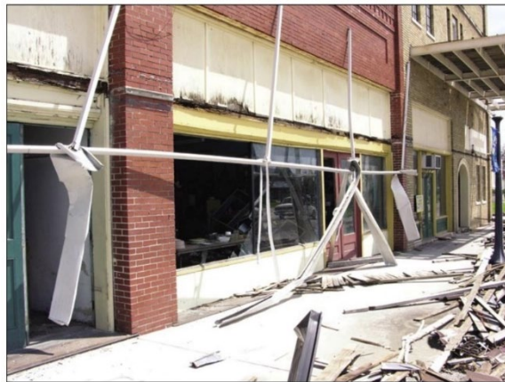
Figure 19. Broken glass windows caused by wind-borne debris during hurricane Charley (2004) in Wauchula.
