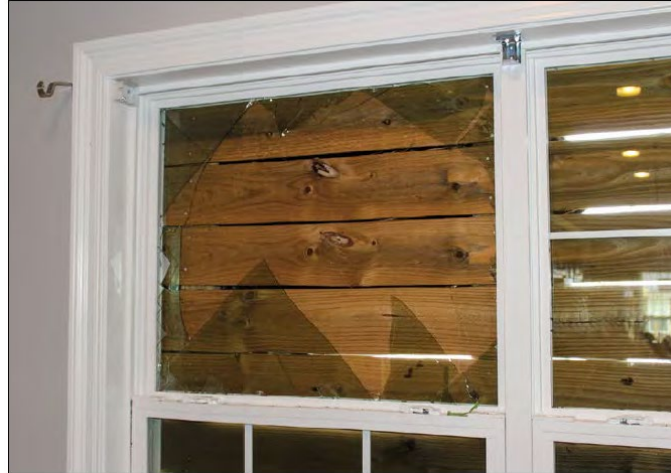
Figure 32. Glazed opening damage caused by an asphalt shingle after Hurricane Michael (2018) in a house built in 2012, located in Panama City. Estimated wind speeds (150 mph) exceeded the design wind speeds (126 mph).
