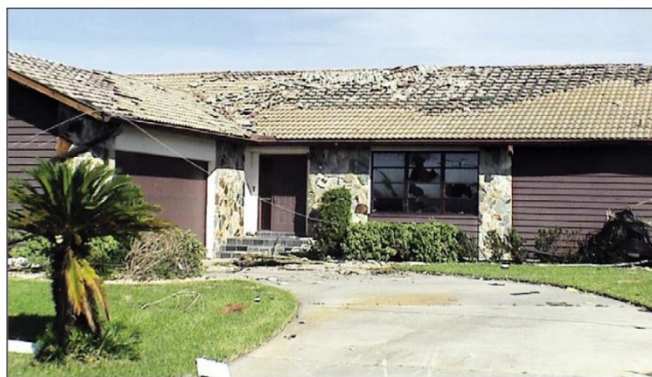
Figure 5. Extensive damage of pre-2001 FBC home. Broken windows caused by wind-borne debris during Hurricane Charley (2004).
