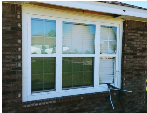
Figure 38. Damage to a window in Panama City during Hurricane Michael (2018). House was built between 2010-2019 and located 3.39 miles from St. Andrew Bay. Estimated wind speeds (129-150 mph) might have exceeded the design wind speeds (135 mph).
