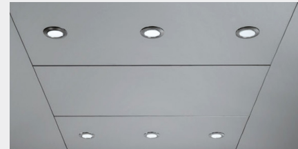
Ceiling lighting — Standard LED round spot downlights*
