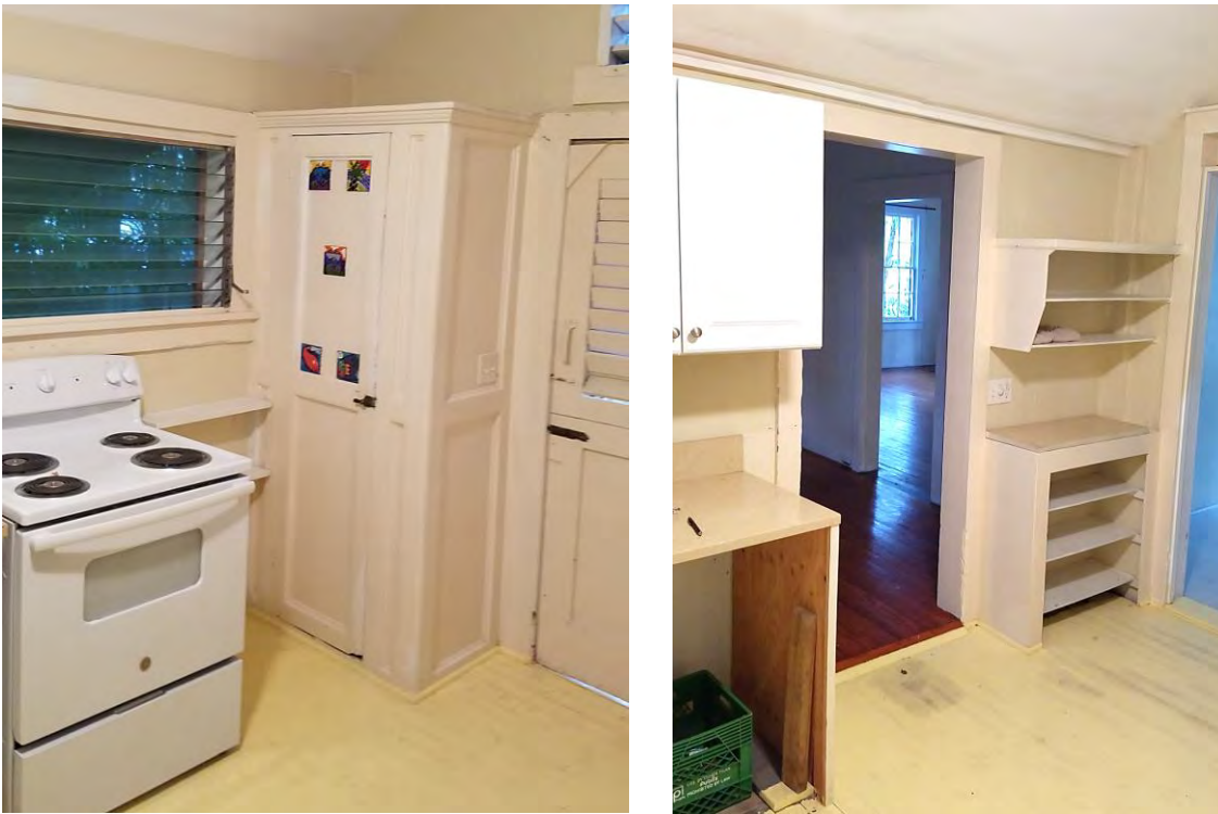
Pantry (left) and shelves (right) in the kitchen of 624 White Street. The shelves were almost certainly installed for Bishop and Louise Crane. (Bender & Associates)
