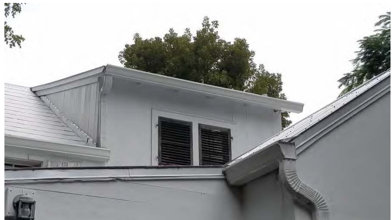
This view of the 2 nd floor dormer shows the aluminum ogee gutters and square downspouts on the house. These gutters and downspouts are not appropriate for the house.
