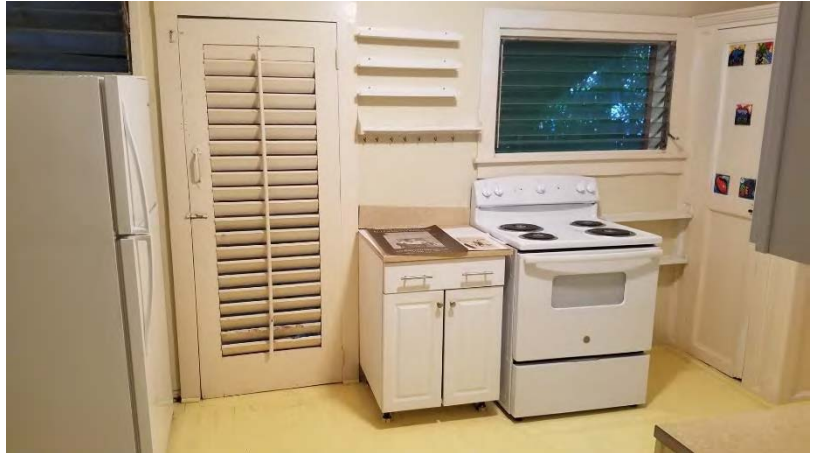
The two aluminum jalousie style kitchen windows at the south façade. The windows should be removed and replaced with painted wood windows.
