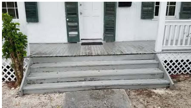
The painted wood main stair leading from grade to the front porch.
