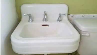
Detail photo of the lavatory at the 2 nd floor bathroom. This fixture likely dates to Bishop's time, though the fittings have been changed. The adjacent WC is modern.
