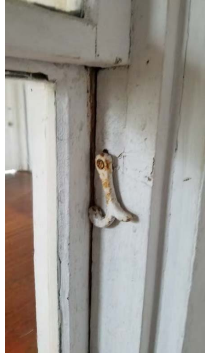
This piece of hardware holds the single hung windows in an open position. It is found on virtually all of the windows.
