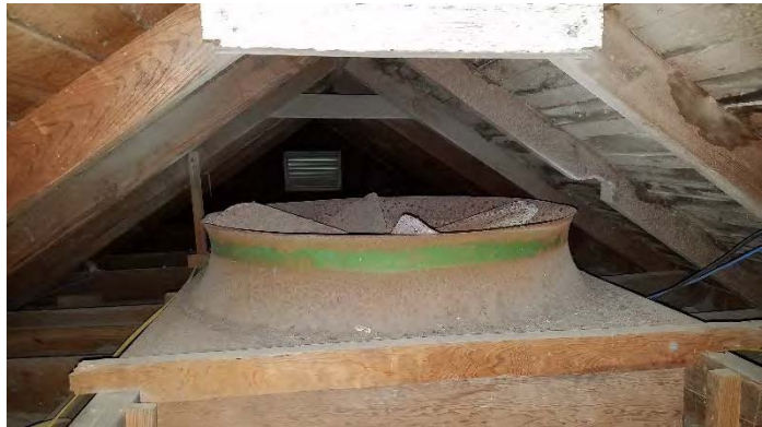
The whole-house fan as seen from the attic. The unit is functional, but very worn. It probably dates from the early 20 th century.
