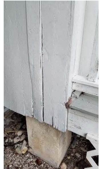
This view of the SE corner of the house shows damaged siding at the base of the building. The front porch can be seen at right.
