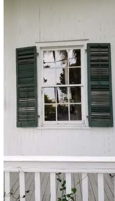
A typical window at the front façade of the house. The windows and the louvered shutters are very significant.
