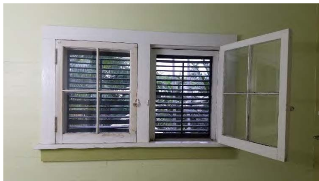
This photo shows the painted wood inswing casement window at the bathroom dormer. The window was operable louvered shutters at the exterior.
