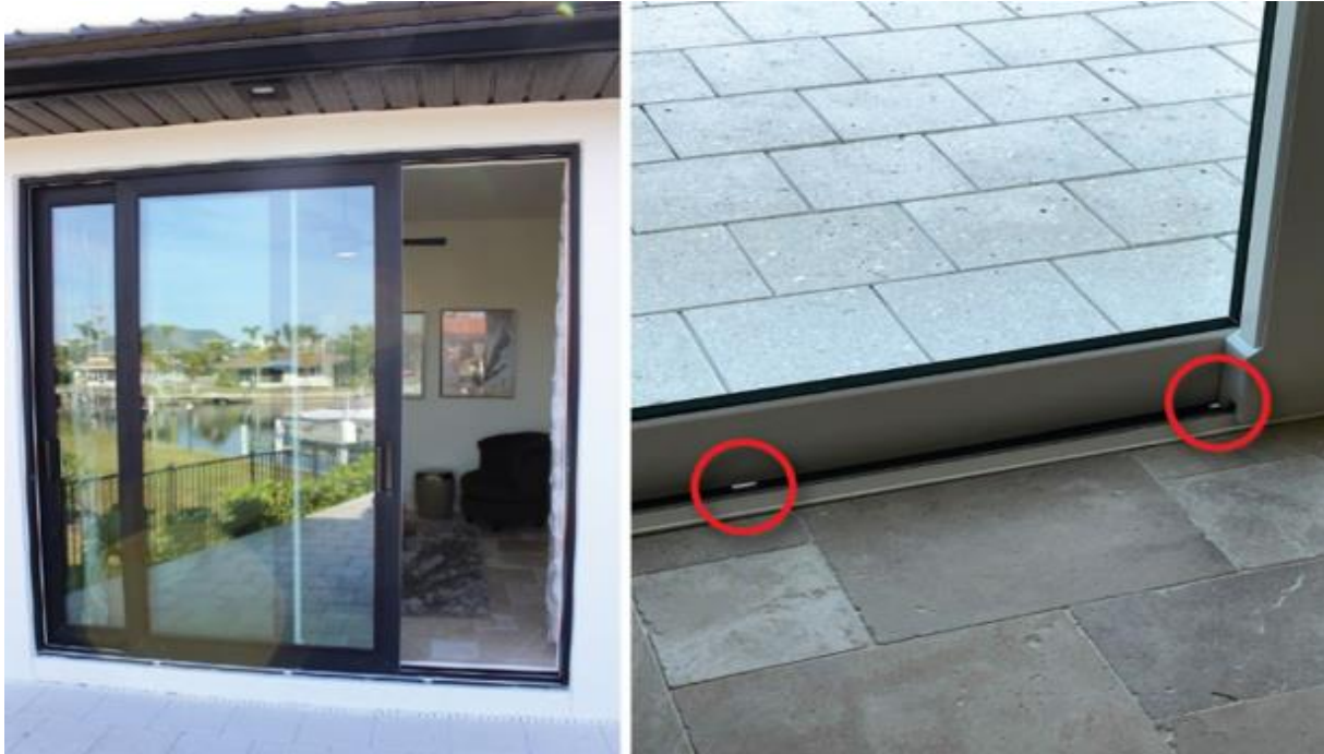
Figure 2 Due to wind-driven rain, a 2021 home with a two-panel sliding glass door suffered severe water intrusion (the two red circles indicate weep holes that allow water to depart). DWS is 11 mph, and EWS is 130 mph. (Punta Gorda)
