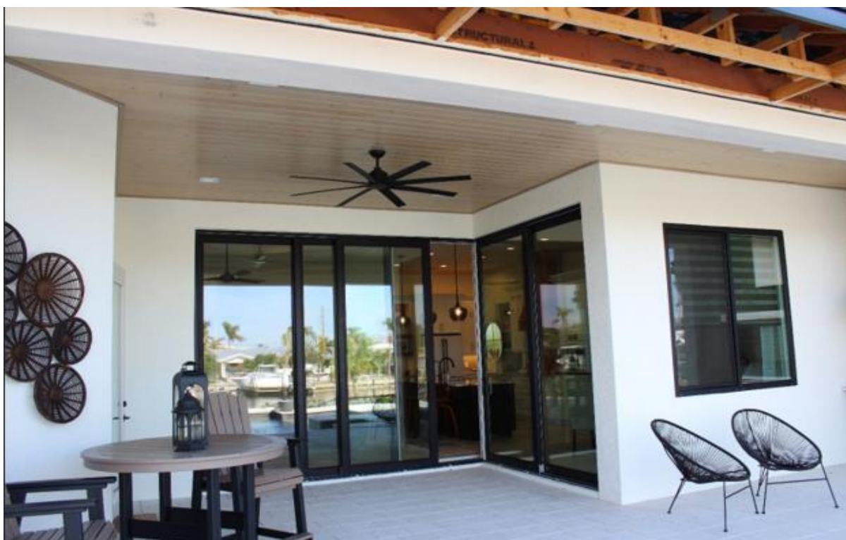
Figure 1 Significant water intrusion occurred in a 2021-built home with two and three panel SGD (EWS = 130 mph; DWS = 151 mph) (Punta Gorda)
