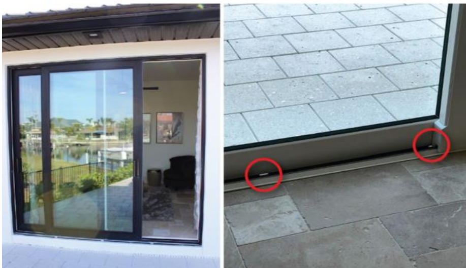
Figure 2 Due to wind-driven rain WDR, a 2021 home with a two-panel sliding glass door SGD suffered severe water intrusion (the two red circles indicate weep holes that allow water to depart). DWS is 11 mph, and EWS is 130 mph. (Punta Gorda)
