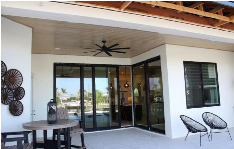
Figure 1 Significant water intrusion occurred in a 2021-built home with two and three panel SGDSDs (EWS = 130 mph; DWS = 151 mph) (Punta Gorda)
