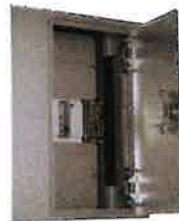
DISCONNECTS ARE PROVIDED
