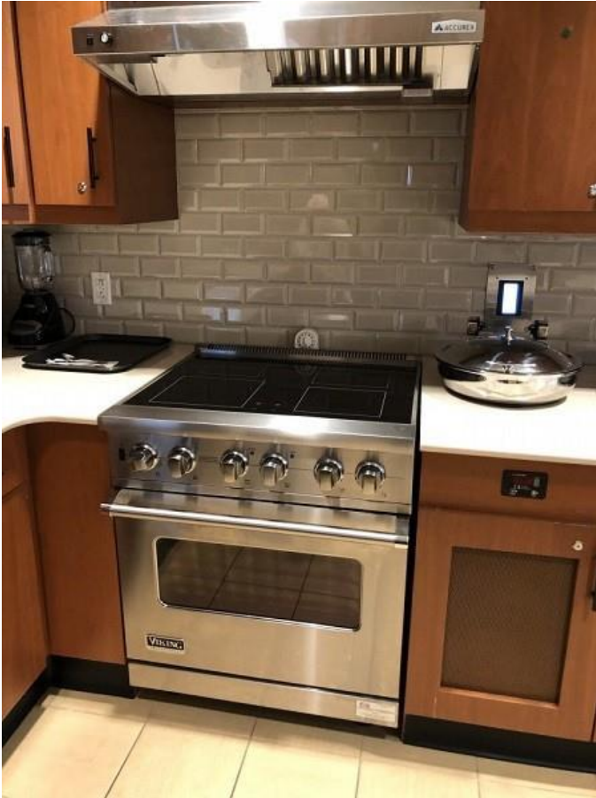
Range with timer control and grease collecting hood.
