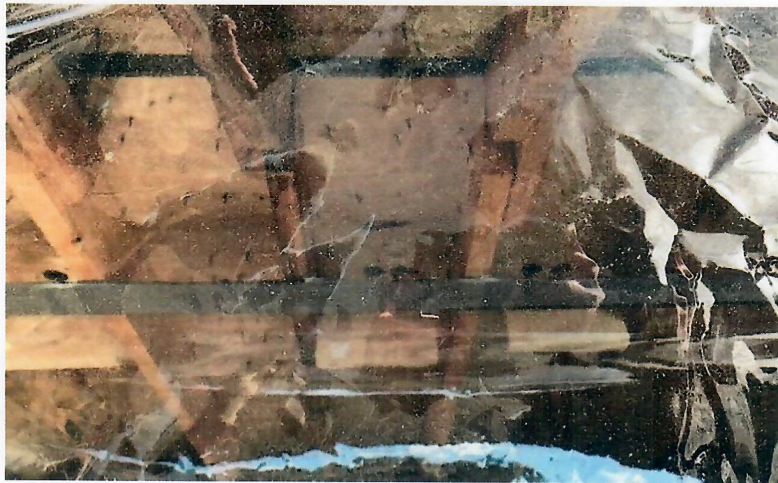
Photo No. 12 Post Test Underside
