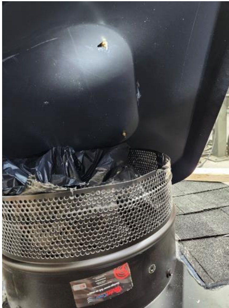
Photo No. 2 AFR SMT PRO-1.3 Failure Photo
