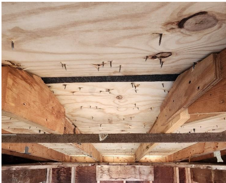
Photo No. 12 Post Test Underside
